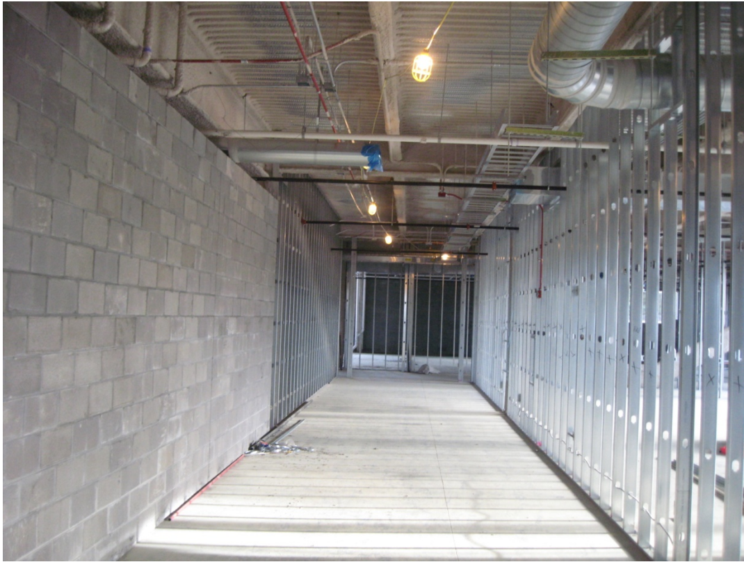
NE Building first, Second, Third and Fourth Floor Electrical, Plumbing and Mechanical Rough-in is Ongoing
