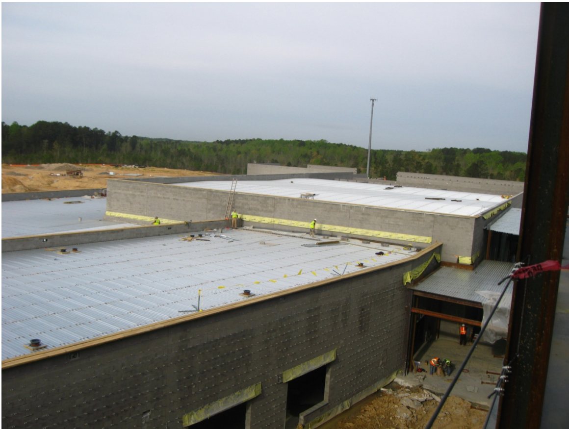
Wood Blocking @ the Roof Parapets are Ongoing Installation of the Roof Drains are Ongoing
